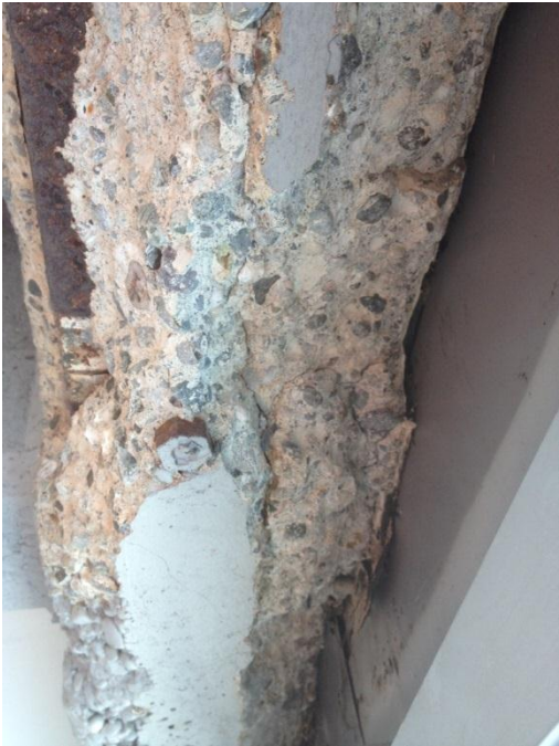
6. View of Bottom of Beam Showing Reduced Section and Exposed Reinforcement
