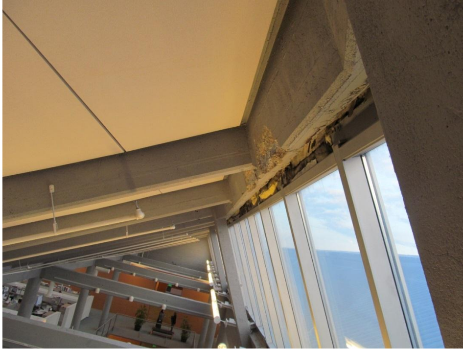
3. Example of Beam Deterioration where repair work was performed ( loose concrete was removed and reinforcement was coated )
